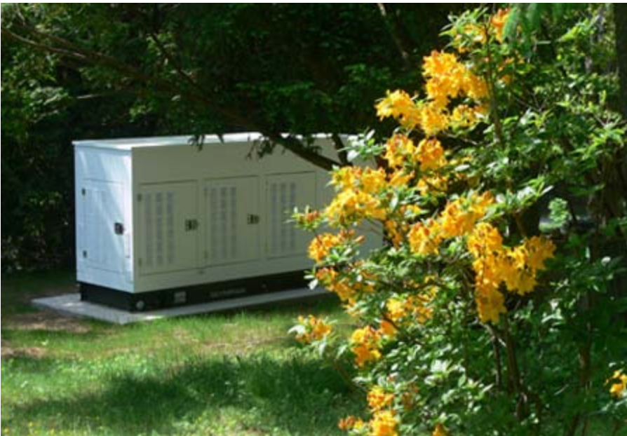
Reliable Power - A new Retreat Center generator is now up and running. It will immediately take over if a power outage occurs, providing sufficient electricity for all the facility's needs, including lights, heat and hot water, and communications.
