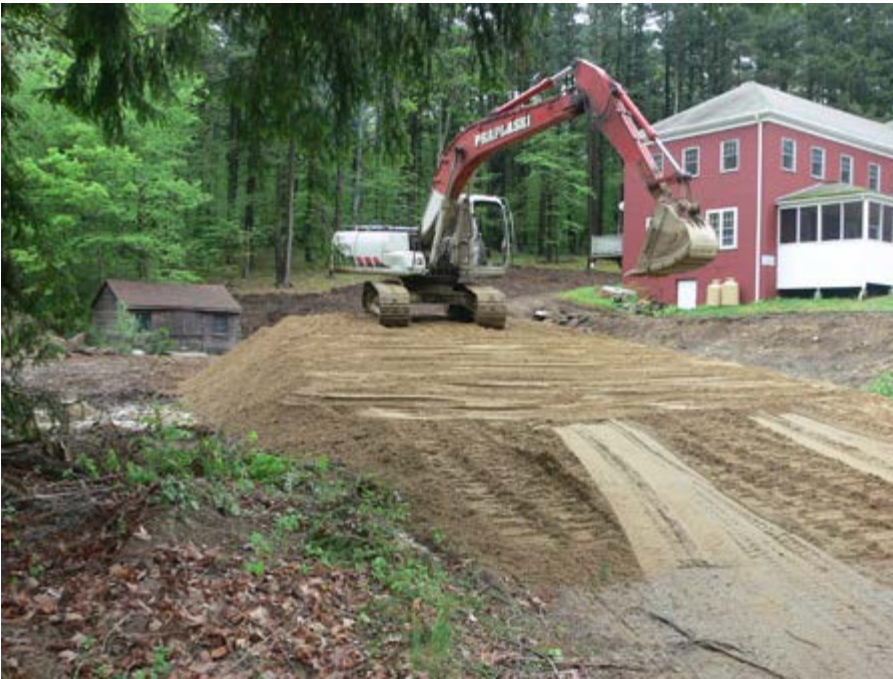
Building up the foundation for a new access road on Retreat Center grounds. This will serve for dropping off luggage at the new dorm and Annex, as well as for delivery and emergency vehicles.
