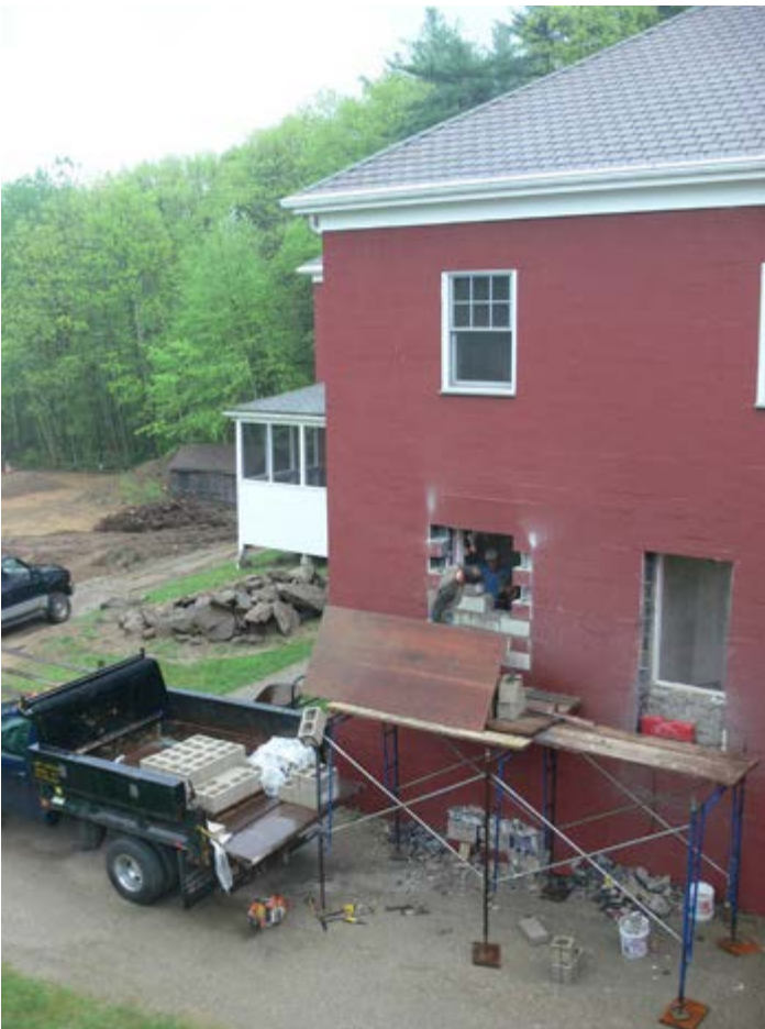
Preparing the Annex for the covered walkway that will connect all three dorms to the rest of the Retreat Center facility.
