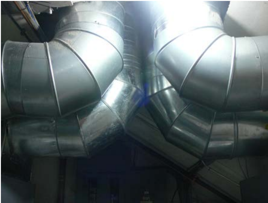
Behind-the-scenes view of ducts that will provide fresher air in the Retreat Center meditation hall.
